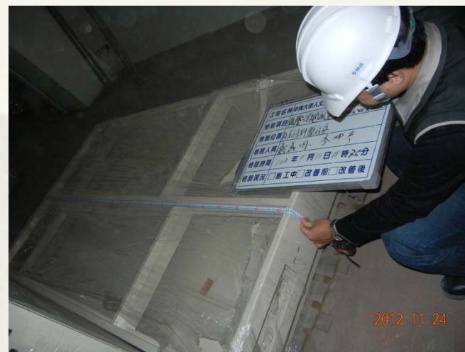
低壓配電盤查驗
